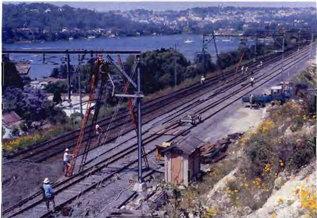
Changing the alignment from the northern approach to the old bridge to the approach to the new bridge in November 1972.
