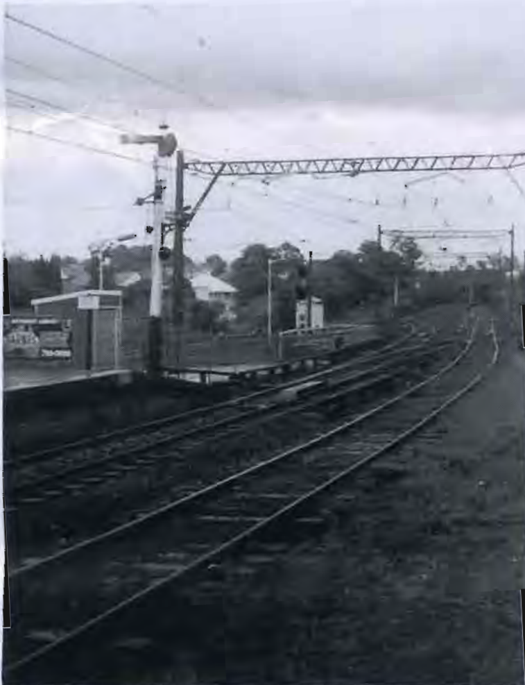
Oatley Station looking north. The Engine Siding is on the right and becomes the Carriage Siding beyond the crossover. Note the small shunting signal on the nearest signal post that directs trains onto the Carriage Siding. RRC305412
