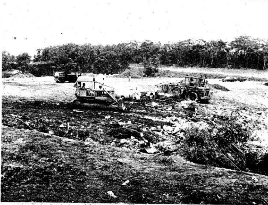
BULLDOZERS dump garbage in the upper reaches of Lime Kiln Bay.
